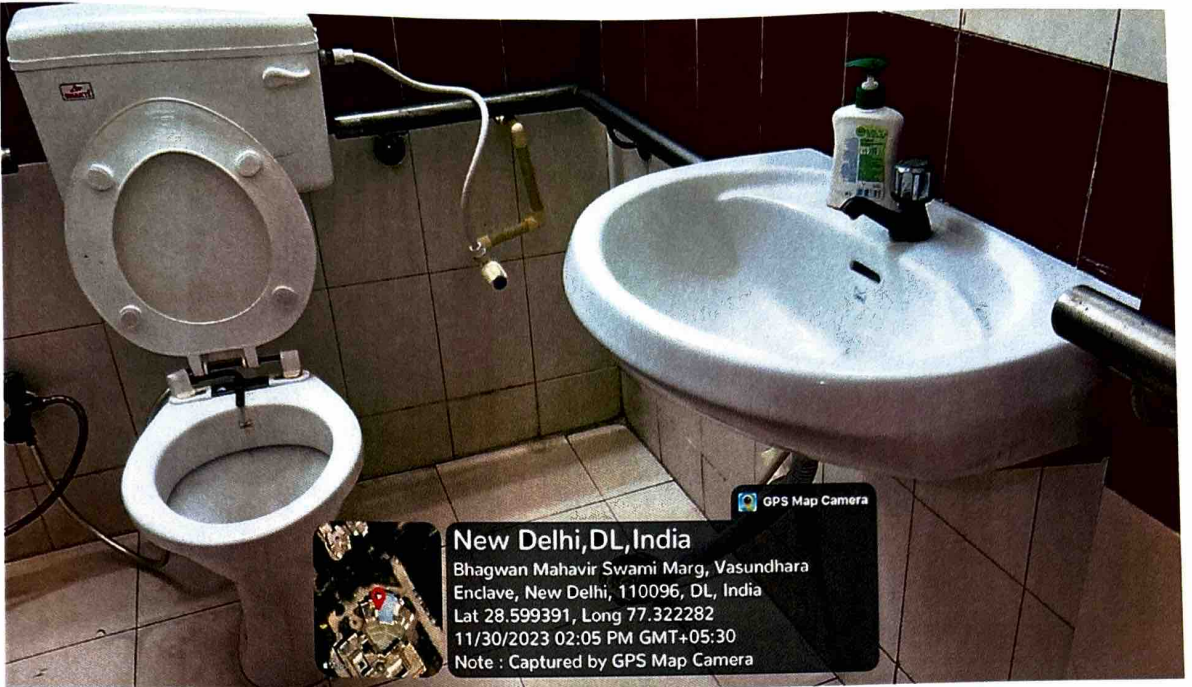
Disable friendly toilet arrangement
