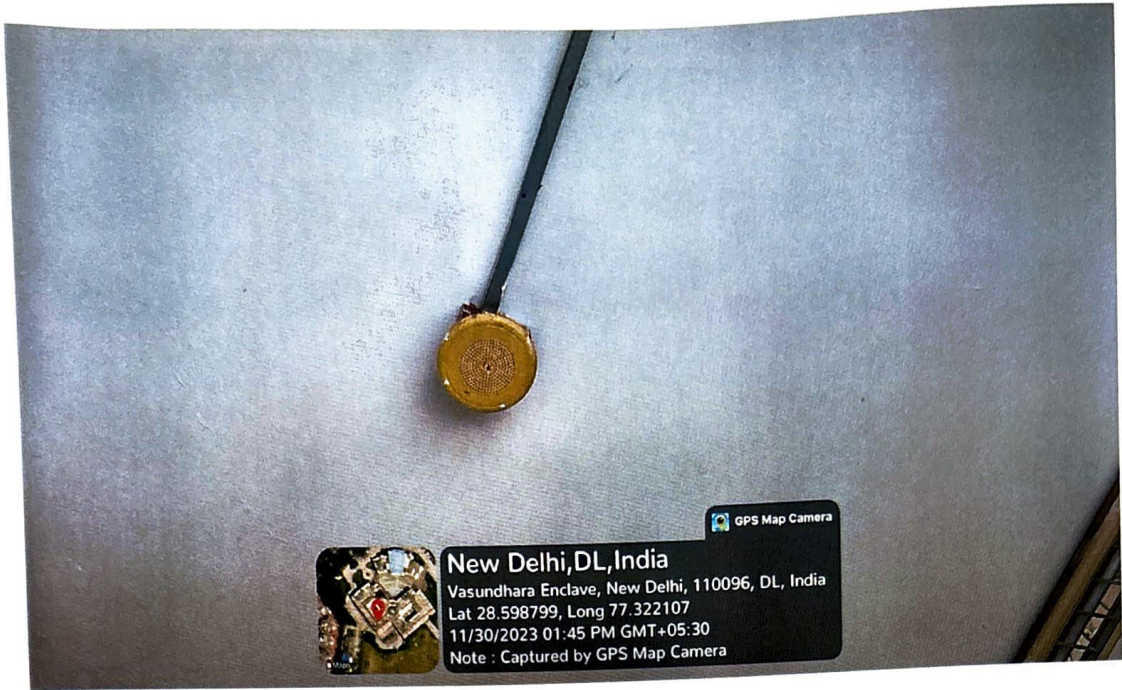
Fire alarm sprinkler system
